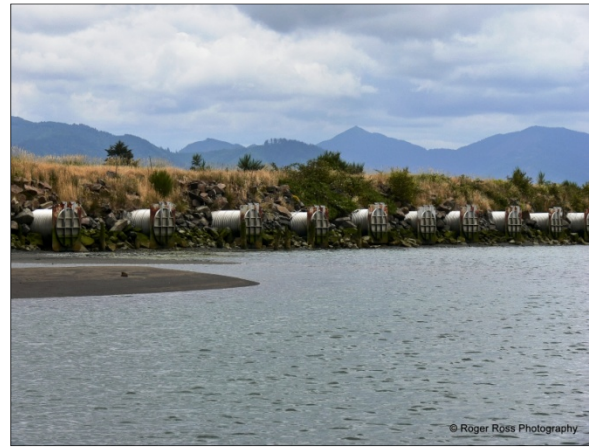
Bank of 10 Tidegates in South Levee (tidegates and levee will be removed to restore full tidal inundation)
